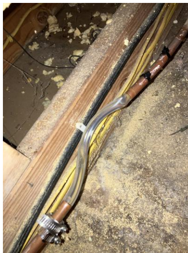
The attic line above the closet after temporary repair
